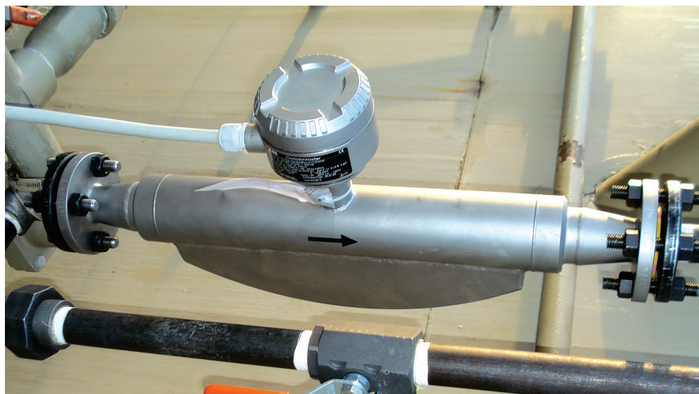
Figure 3. ABB's recently introduced CoriolisMaster flowmeter installed in an upstream oil/gas application, measuring the flow of oil and water with significant gas entrainment.
